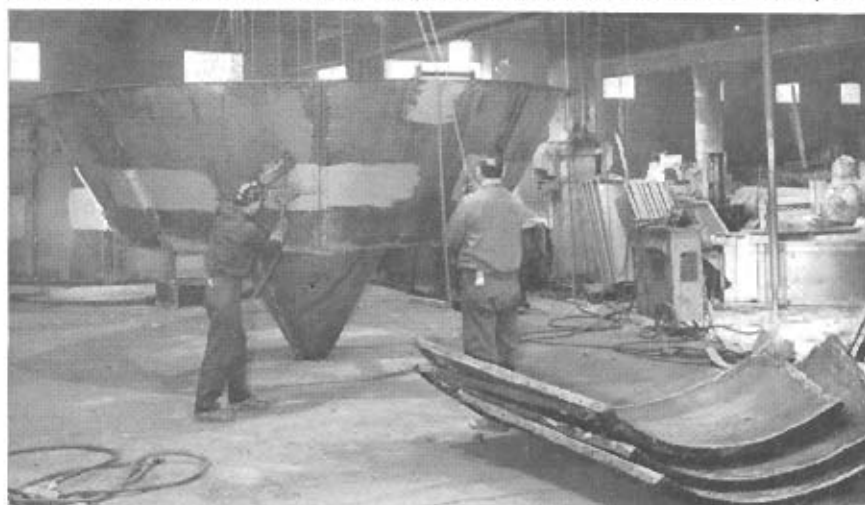
Workman at the Sturtevant Mill Company's plant in Dorchester are shown working on the fabrication of the cone section of a 16-foot air separator which is under construction at the plant.
